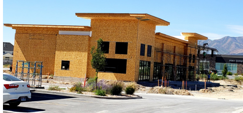
A Mexican restaurant is planned for another retail building under construction in City Center.
