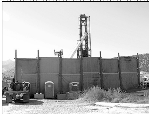
Drilling is underway on the city’s well #4 in the Kiowa Valley area (see news notes pg. 3).
