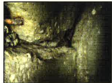
Cracked concrete sewer line
