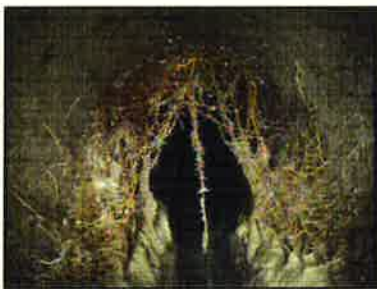
Root penetration into concrete sewer line
