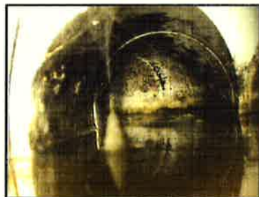
Belly in PVC sewer line
