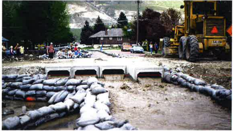
Figure 4 Sandbagging in Provo during the 1983 floods
