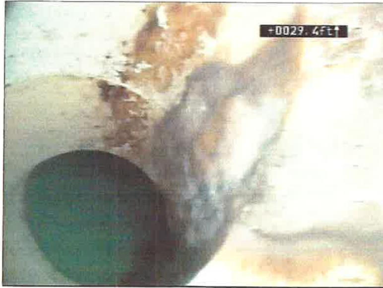
Photo: 410_2A 29.4FT, service connection with grease, at 02 o'clock
